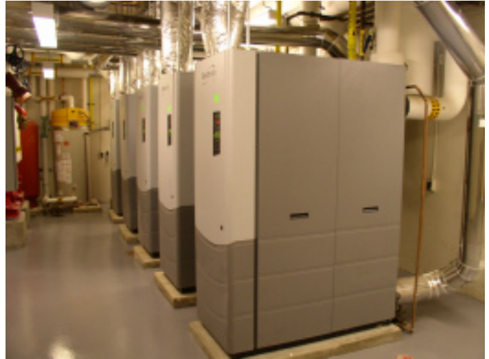
Five 2 MBtuh capacity Aerco Benchmark™ boilers at CC&SU central plant
