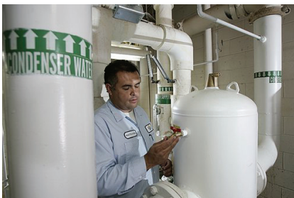
Tony Regalado taps water from the 4900 Series Air Separator
